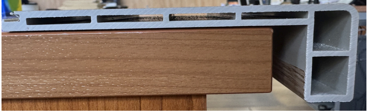
Incorrect installation — unsupported overhang beneath the stair nose.
